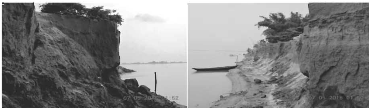
Image: Bank erosion Boralimari.
